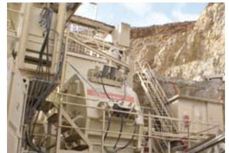
Stationary : Primary NP1415 Impact Crusher fully hydraulic equipped.
